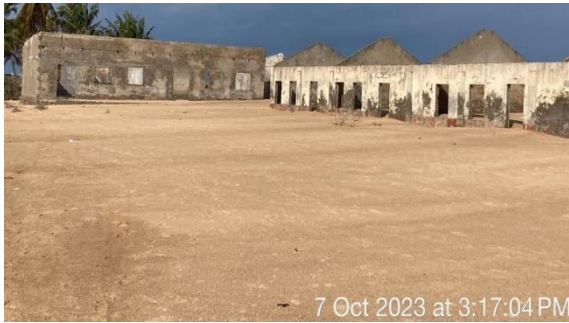
Figure 7-19 - Homes Impacted by Sea Erosion and Lagoon Floods
